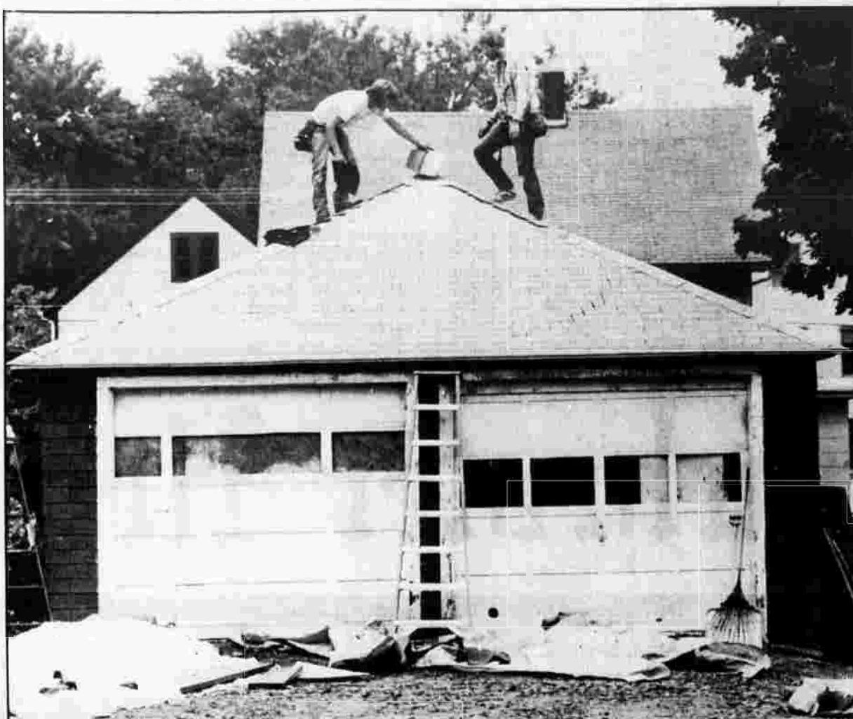
REPAIR WORK — Matt Schrag of Glastonbury, left, and Paul Marella of 0133 Jordt St. repair the roof on a garage on Bissett Street Tuesday. The men worked on the roof despite a light rain.
